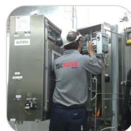
Service on site per TOC in cabinet EEx p
